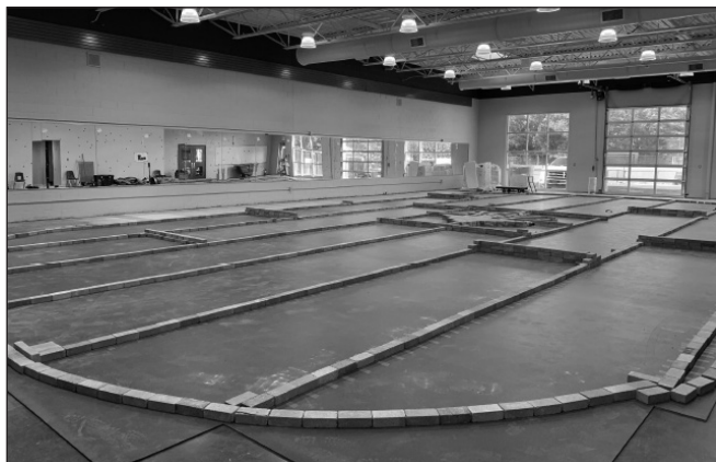
The new sports flooring has been installed in the new Weight Room. New weight equipment will be installed in the next few weeks
