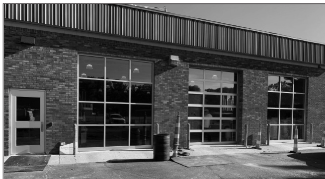
The new Fitness Center glass walls and overhead door are complete and will let in a tremendous amount of light!
